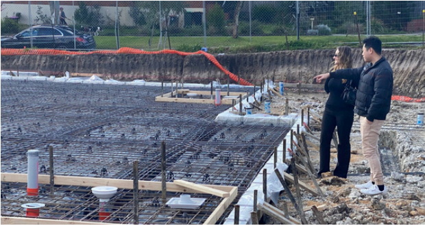
Vic and Chelsea on the site of the newest Out of Home Care project, prior to the first concrete pour.
