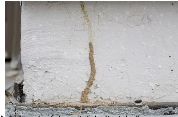
An example of a termite "shelter tube"
