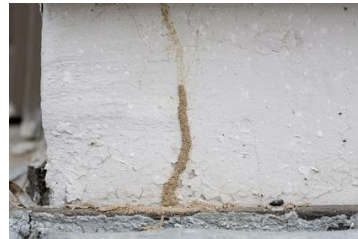
An example of a termite "shelter tube"
